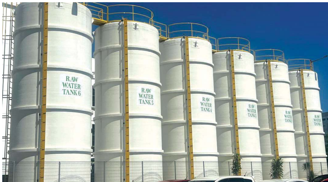
Water storage tanks at Penang P13 (Malaysia)
