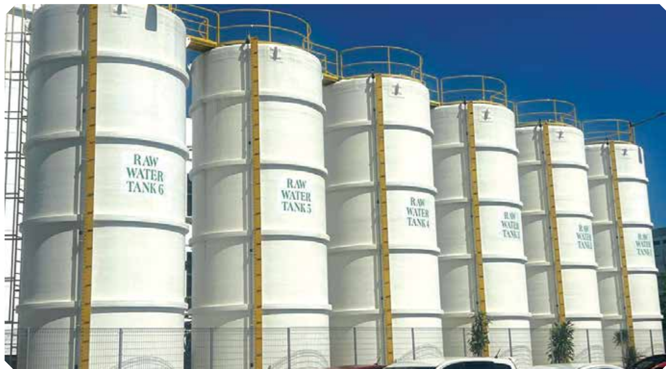
Water storage tanks at Penang P13 (Malaysia)
